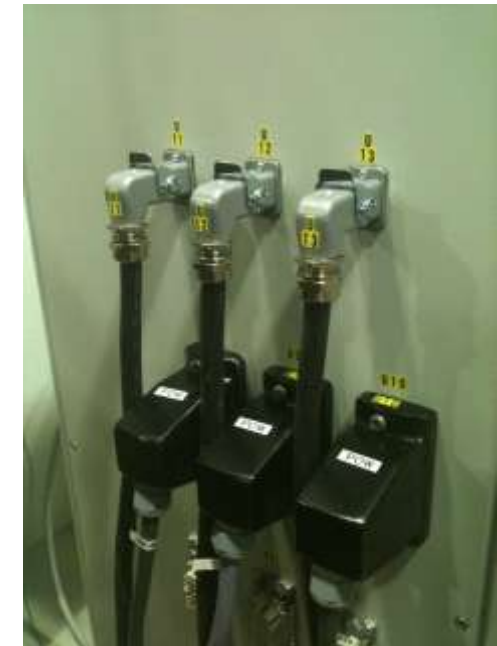
Prefixed cables between units
