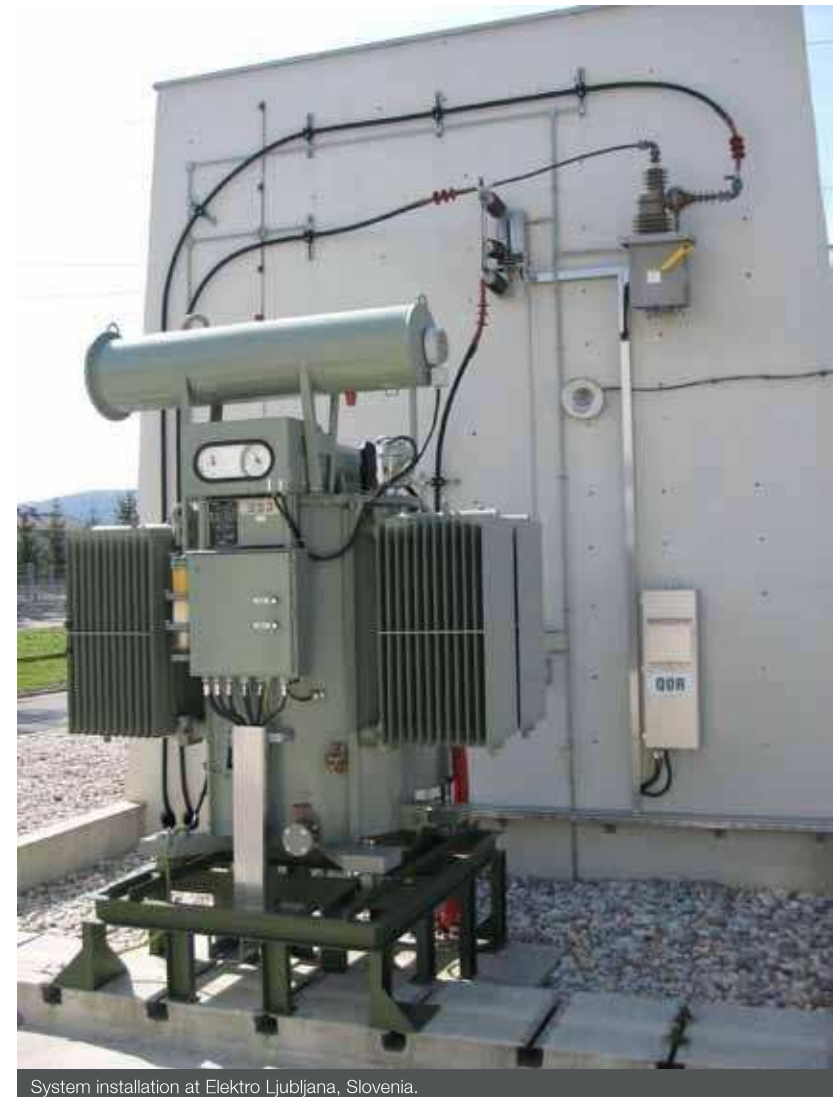
System installation at Elektro Ljubljana, Slovenia.
