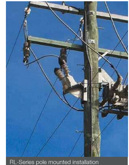
RL-Series pole mounted installation
